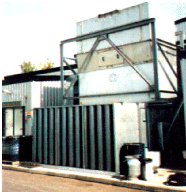
Large stainless steel silencers on a cooling tower which was just one of the 105 sources on this site.
